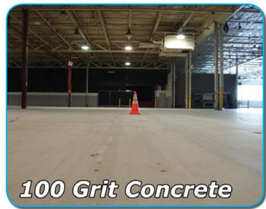
FIGURE 2-A: AFTER 100 GRIT CONCRETE PREP TOOL. YOU WILL NOTICE ANY DIPS IN THE FLOOR THAT MIGHT NEED ANOTHER PASS OR TWO.
