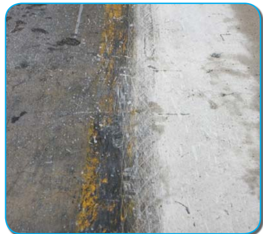
FIGURE 2-B: UNIFORM WHITENING ON THE CONCRETE WILL BE VERY NOTICEABLE. IF NOT - CONTINUE PROCESS TILL FLOOR IS UNIFORM.
